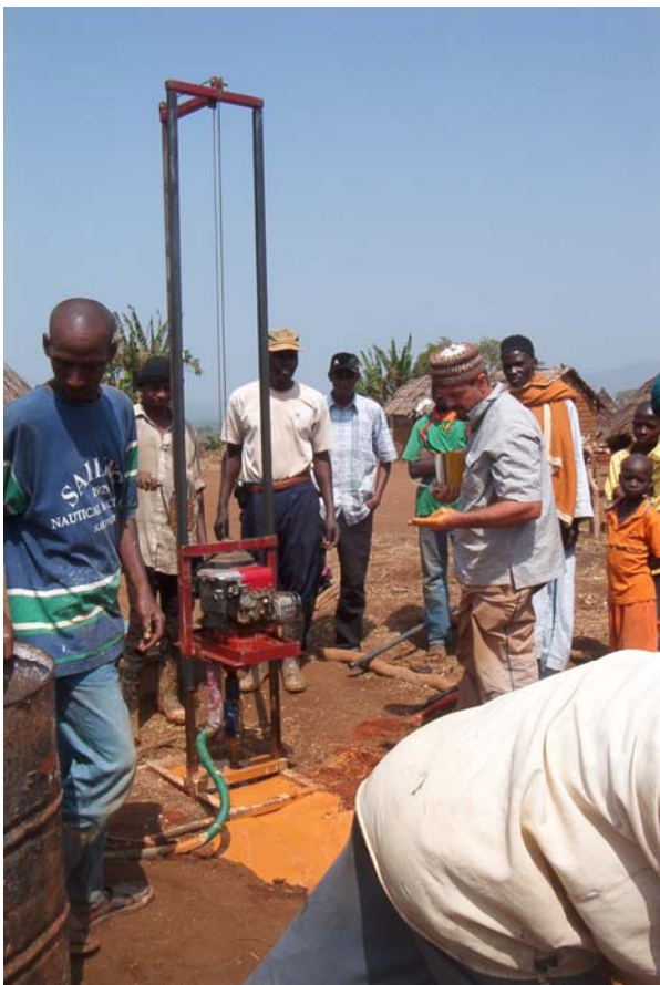
TEST DRILLING AT A PROPOSED HAND DUG WELL LOCATION TO DETERMINE DEPTH TO WATER
