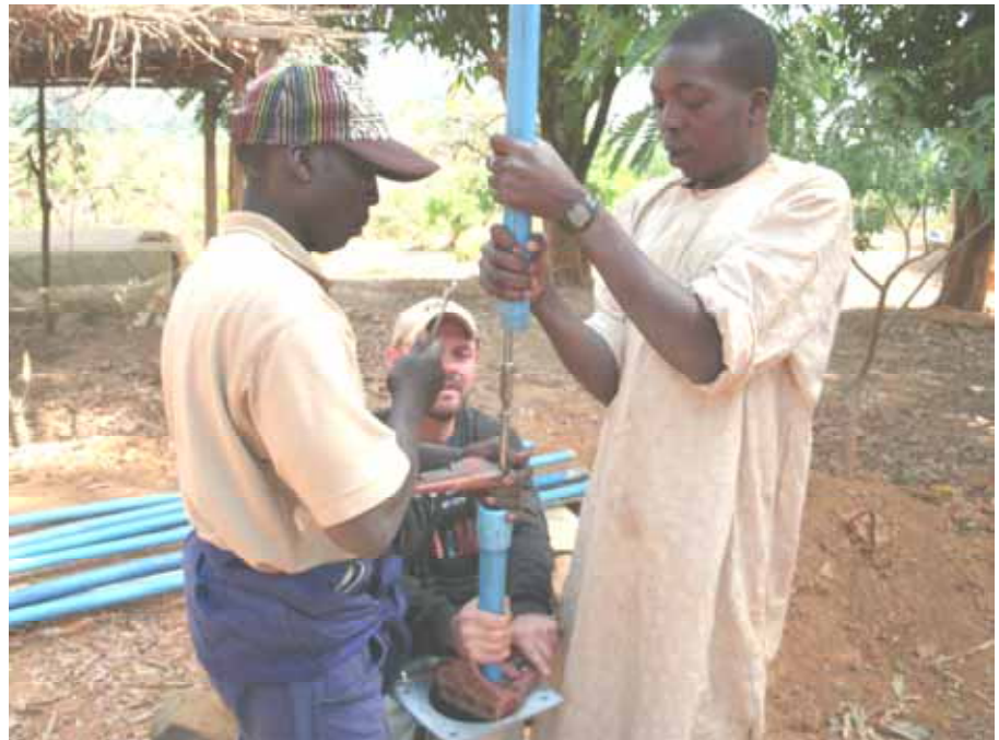
Chad works with two technicians to install the recovery pipe and steel rods for the manual pump. This well will provide clean water for at least five different “compounds” and over twenty people in our area of the community.
