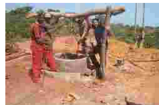
Chad hangs with the crew as excavation continues in a hand dug well
